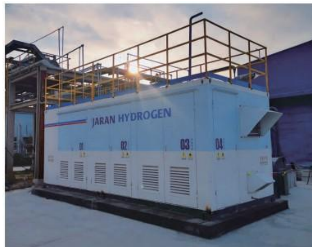
Modular directional impurity removal-hydrogen mother station
