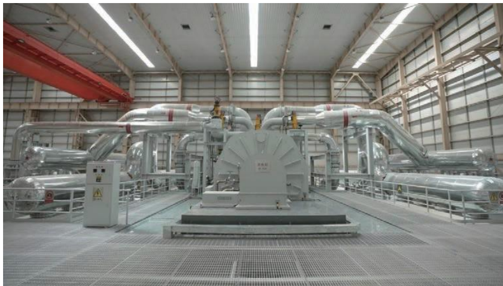
Field equipment diagram of compressed air energy storage system of the company
